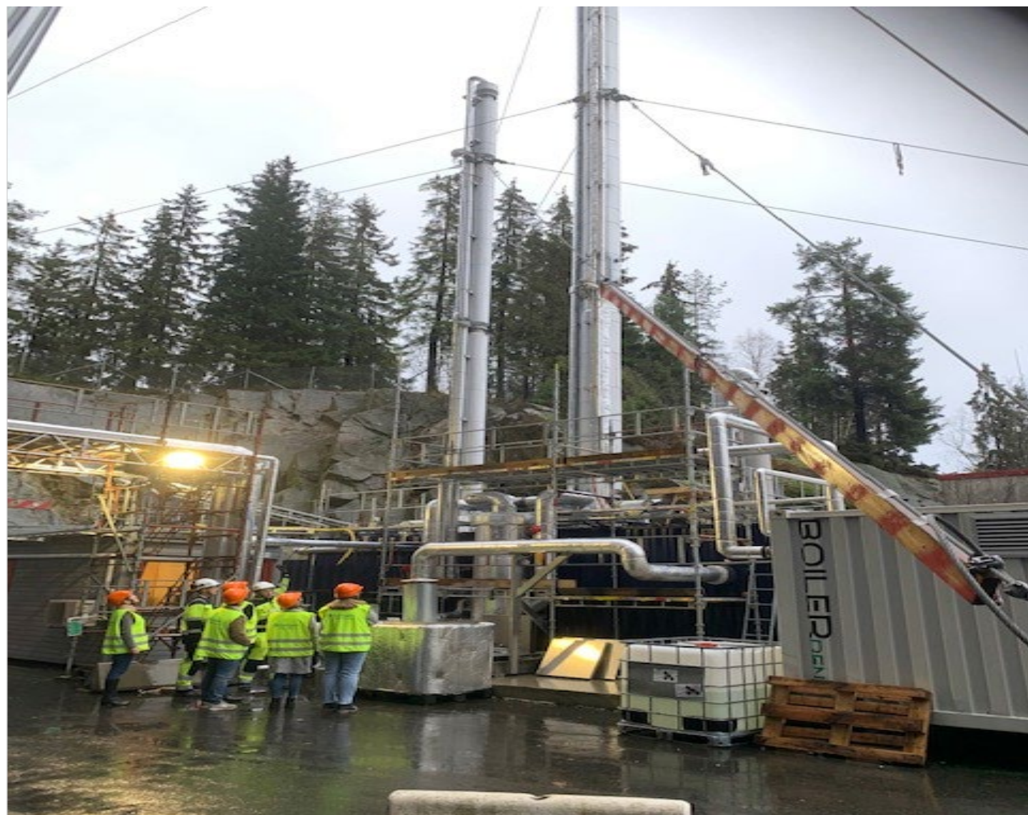
CO 2 capture pilot at Fortum Oslo Varme AS, Klemetsrud
